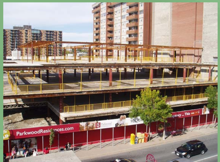
Figure 1, This commercial building was stripped back to its structural frame to be used to create new apartments in Oshawa.
